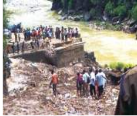
Fig. 1.51: Bridge washed off due to landsliding
