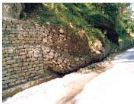
Fig. 1.61: Poor maintenance of mitigation measures causes failures
