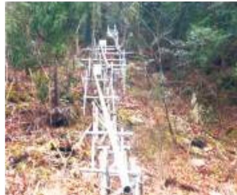
Fig. 6.4: Piped Wire Extensometer for measuring slope displacement
