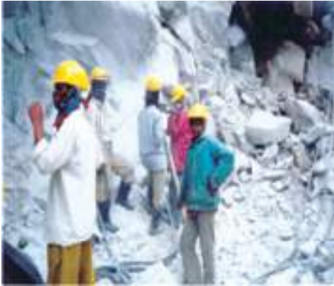
Fig. 1.20: Blasting in road construction leads to landslides
