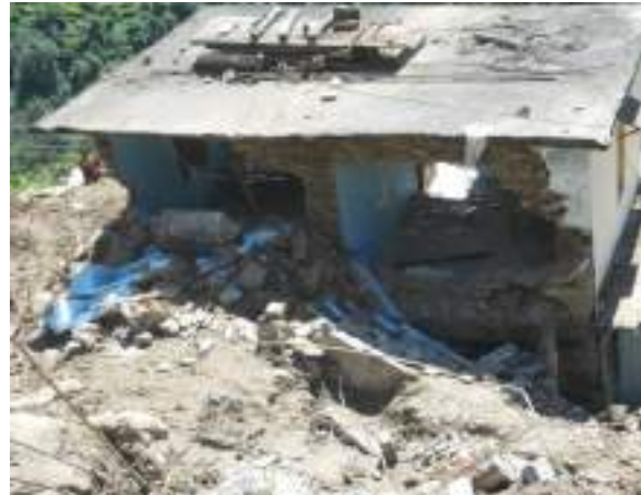
Fig. 36. View of the damaged house.
