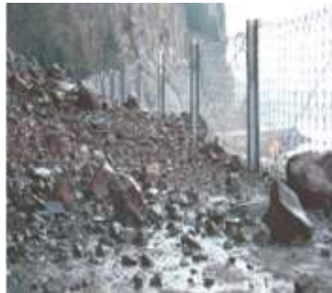
Fig. 7.56: Net Fencing to avoid the impact of sliding on road and traffic
