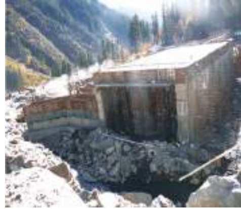
Fig. 7.38: Snow Gallery to avoid avalanches and debris flows along roads and facilitate traffic movement
