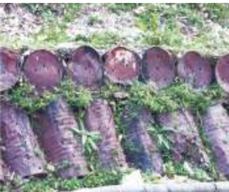
Fig. 7.23: Empty bitumen drums filled with debris acting as retaining wall
