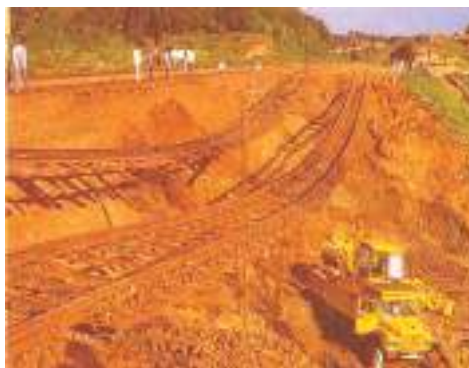
Fig. 1.59: Railway track damaged due to landslides
