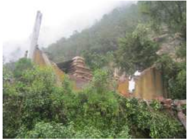
Fig. 11. Damaged food grain storage facility at Bamankholi.
