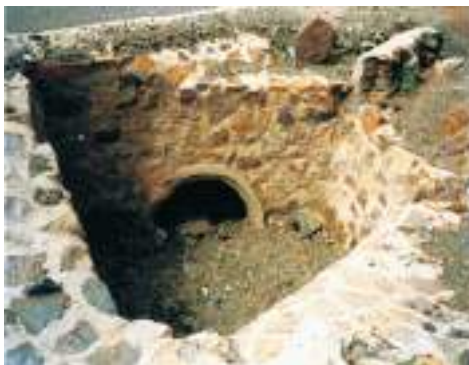
Fig. 1.24: Ill-maintenance and clogging of drainage culverts results in damages
