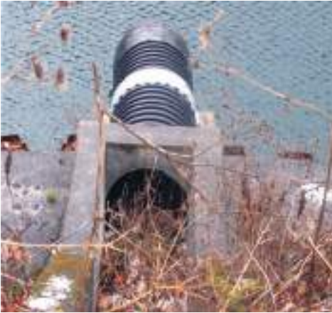
Fig. 7.7: Flexible drain pipe system used to dispose off water responsible for triggering and promoting landslide
