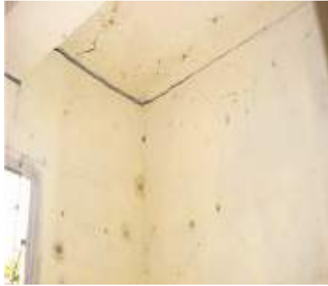
Fig. 1.33: Opening between wall and roof due to differential settlement
