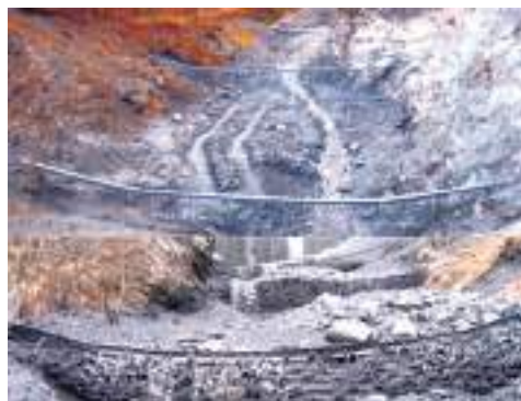
Fig. 1.55: Net barriers to reduce the impacts of debris flow, need proper maintenance
