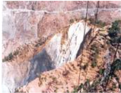
Fig. 1.41: Stability of towers affected due to its proximity with slide
