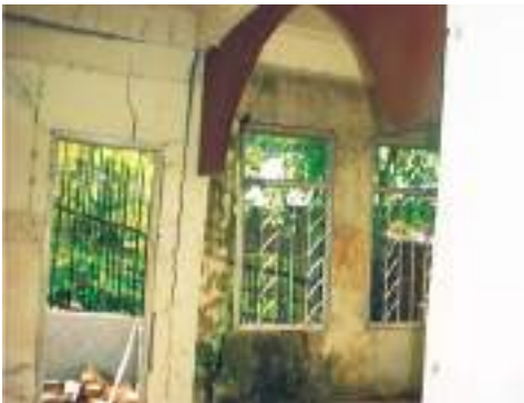
Fig. 1.34: Cracks appear close to doors and windows in a building
