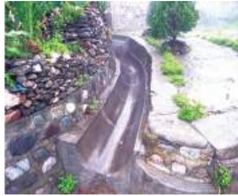
Fig. 7.16: Well lined surface drains at landslide site
