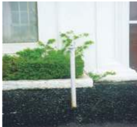
Fig. 6.8: Peg markers used for monitoring slope movements
