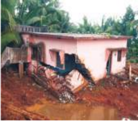
Fig. 1.38: Building gets damaged posing risk to residents
