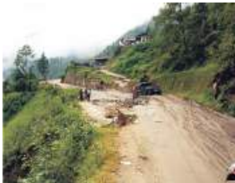
Fig. 1.49: Subsidence causing differential settlement and damage to road
