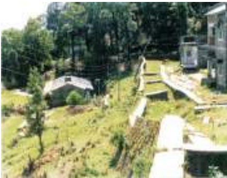
Fig. 1.28: Retaining walls get de-aligned due to landsliding
