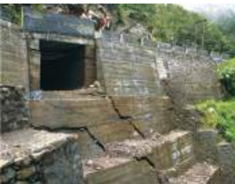
Fig. 1.60: Ill-maintained culverts get damaged and cracked
