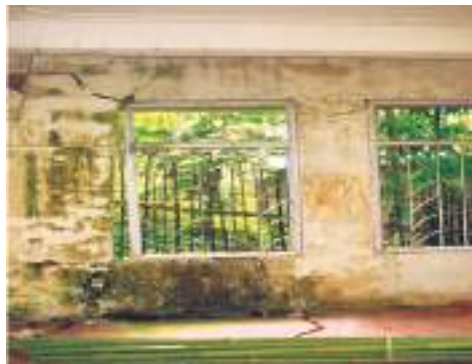
Fig. 1.37: Cracks extend from floor to walls during landslides
