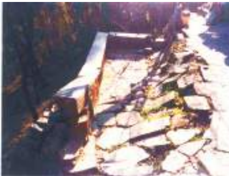
Fig. 1.42: Differential settlement in pavement / floors in houses
