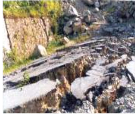
Fig. 1.39: Extensive damages to roads from landsliding
