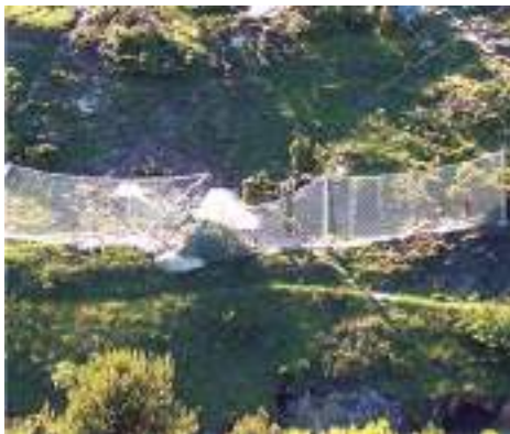
Fig.7.21: Net fencing to hinder rockfall movement on downside
