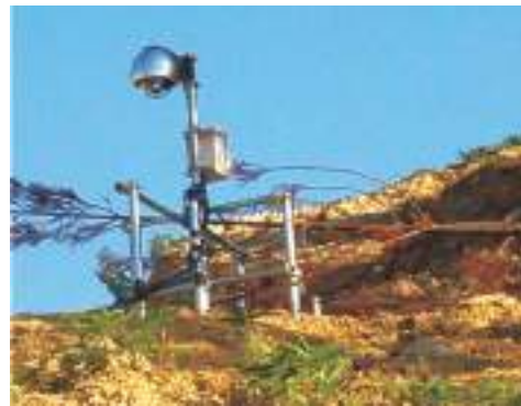
Fig. 6.16: An automated landslide monitoring with recording system
