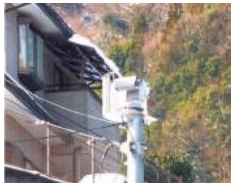
Fig. 6.18: Video Camera and Landslide Alert system with power backup
