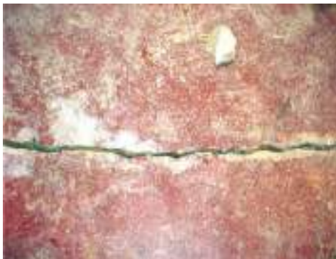
Fig. 1.36: cracks appear in pavement / ground in a house
