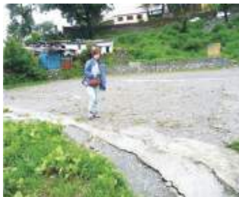
Fig. 7.48: Sealing of cracks with pervious materials beneath the surface and impervious material on top
