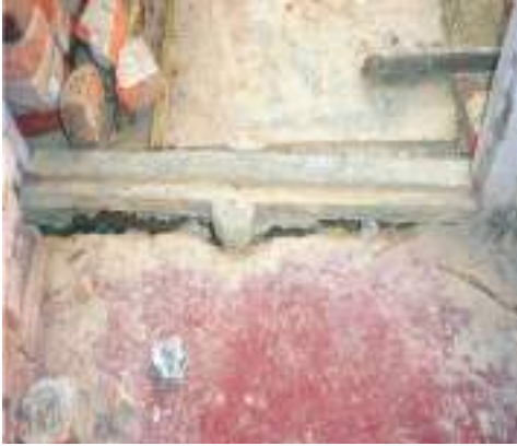
Fig. 1.32: Landslides create gap between door frame and floor
