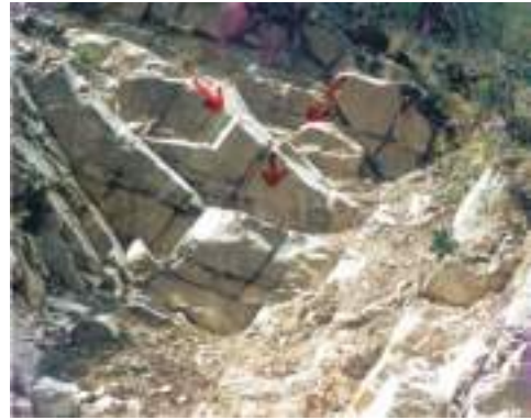
Fig. 1.9: Wedge rockslide due to intersection of two joint planes hading towards valley
