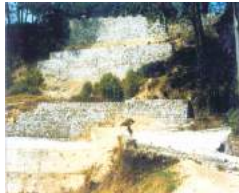
Fig. 7.42: Boulder wall barriers to arrest falling boulders and reduce impact of debris flows
