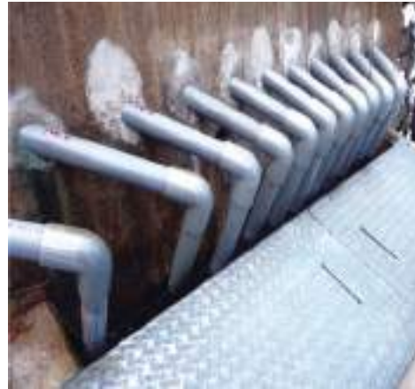
Fig. 7.8: PVC pipes to drain out water from unstable slopes
