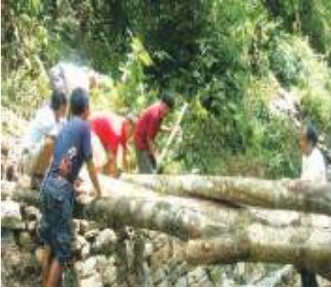
Fig. 8.14: Tree logs being used to make temporary bridge in landslide affected area
