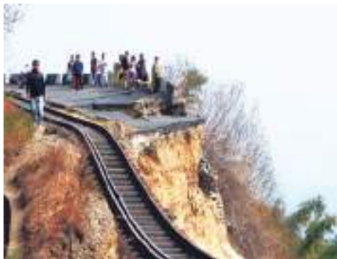
Fig. 1.53: Post-earthquake landslide affects UNESCO heritage toy train track adversely
