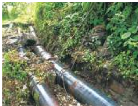
Fig. 1.25: Rigid pipelines and joints get ruptured during landslide and water leakage further aggravates the instability
