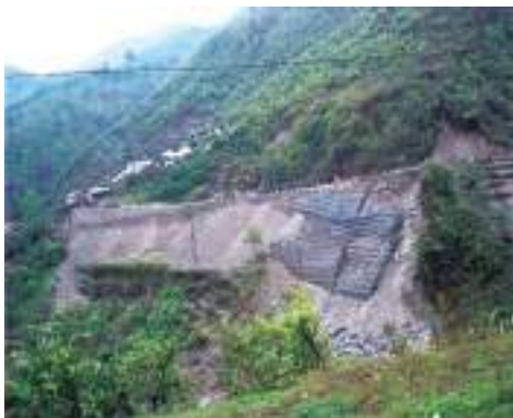
Fig. 8.18: Failure of retaining structures due to weak foundation
