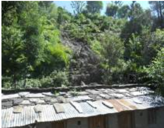
Fig. 41. Photograph showing slight debris flow at backslope of the house.
